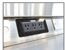
Power feed panels
